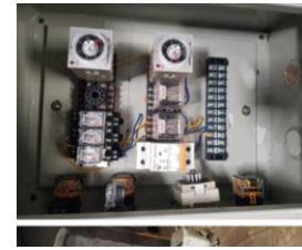
Fig. 6. Filling Machine Control Panel
