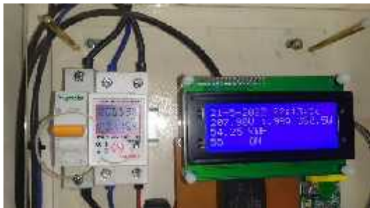
Figure 5. Sensor Testing Process
