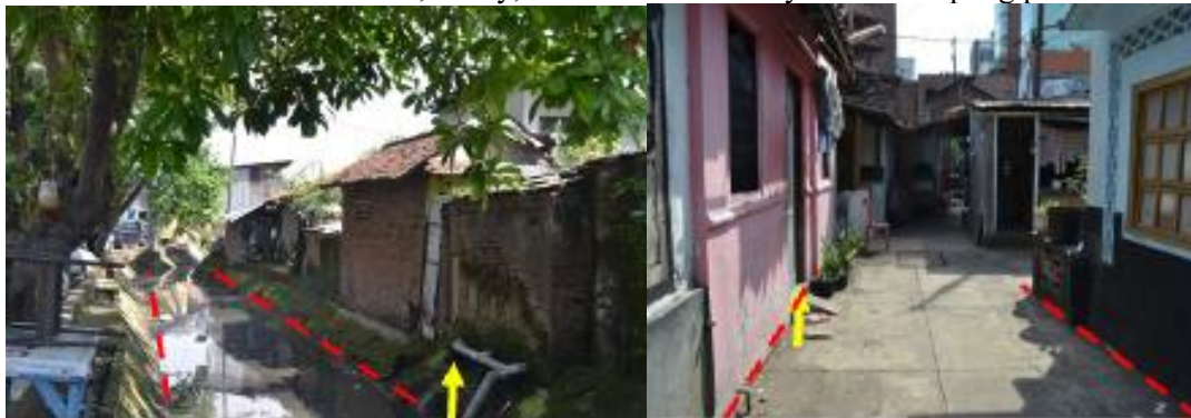
figure 8. drainage conditions and circulation access within Keputran Kampung RW.11
